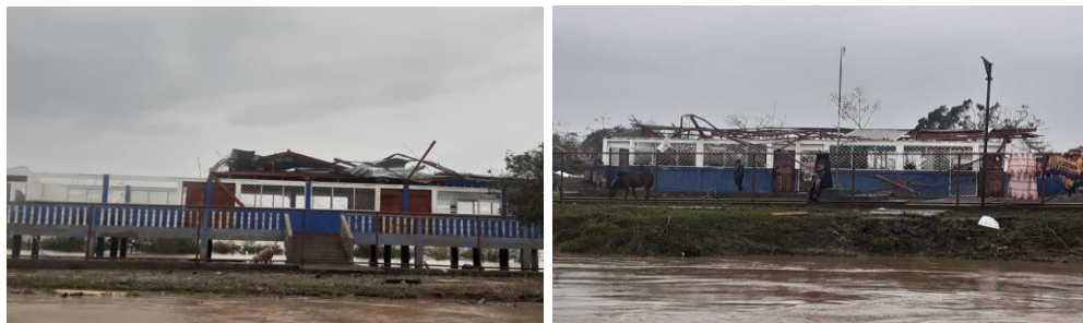
Fig. 1 Schools destroyed by Hurricane Iota in Miskito Indigenous communities in Prinzapolka municipality, Northern Caribbean Coast of Nicaragua, November 2020
